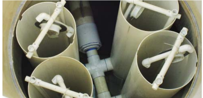
Filter housings were fabricated and assembled before shipping to the tank installation site.
