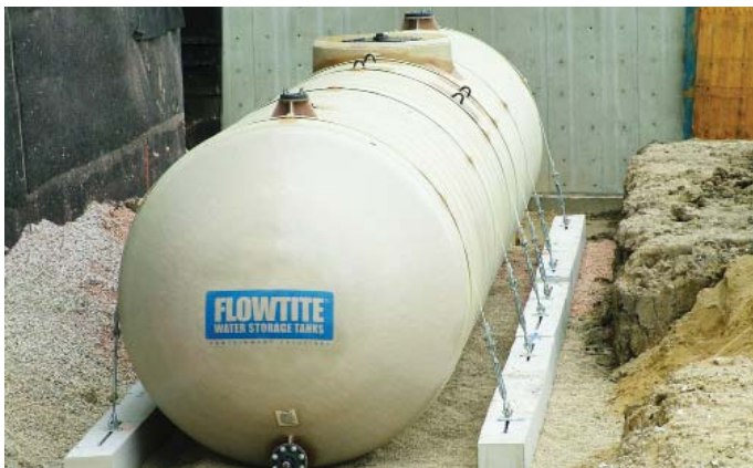
Piping connects to a flanged nozzle on the Flowtite tank to facilitate the transfer of water to the fire protection system.
