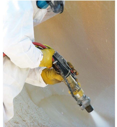
The tank surface is abraded to allow for a strong mechanical bond.
