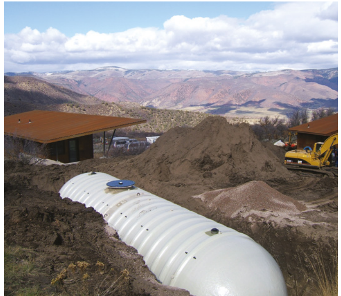
Potable water tanks are frequently used for back-up or emergency water supplies at parks, resorts, rural development as well as heavily populated areas with limited excavation possibilities.
